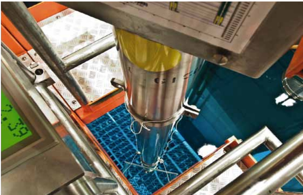
A robotic arm is used to move the fuel assemblies in the spent fuel storage pool.
