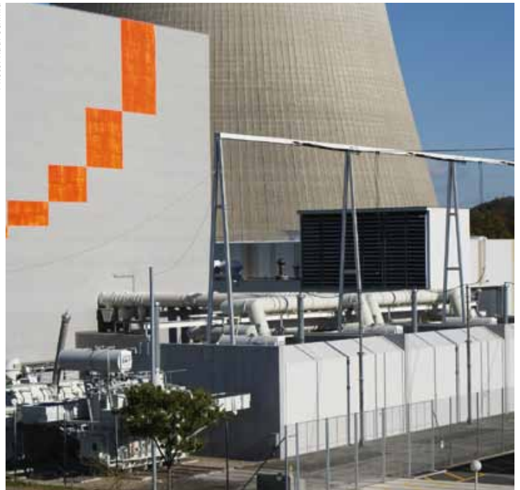
Three transformers form the unit transformer; the fourth one on the left is kept as a standby transformer.
